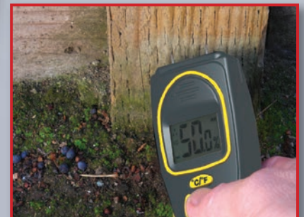
Check wood for dampness or rot
