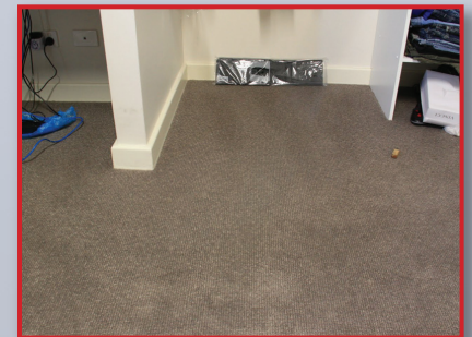
Check for moisture damage up to 2 in. below carpet surface
