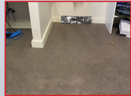
Check for moisture damage up to 2 in. below carpet surface
