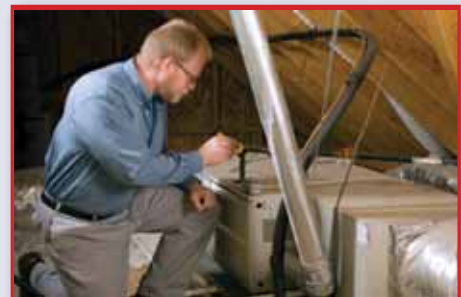
Calibrating HVAC Systems
