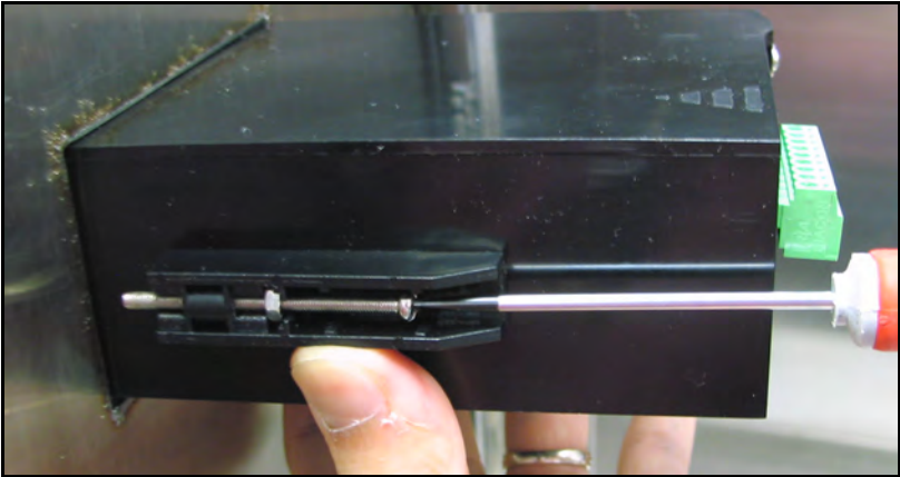
Figure 14: Securing the Single-Channel Hygrometer to the Panel
