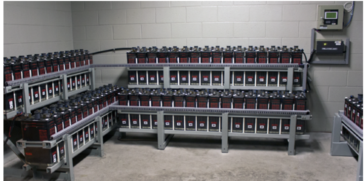
iPQMS Installation on 125VDC Utility Battery System
